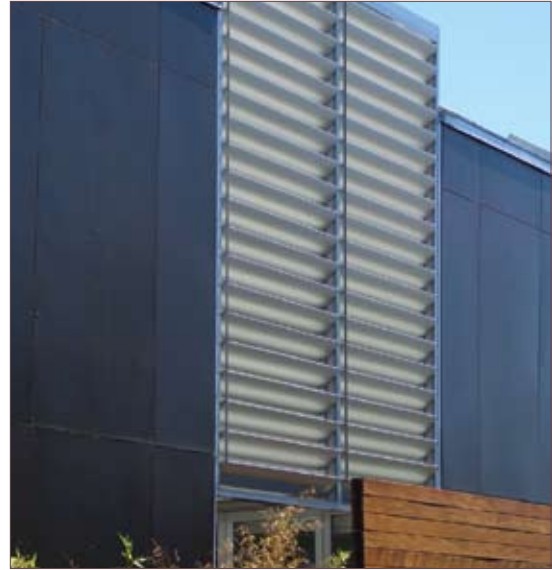
Louvres fixed to the building facade
